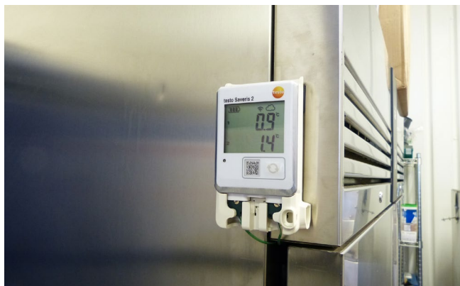
Testo Saveris 2 loggers are used to monitor temperature in refrigerators and a freezer.
